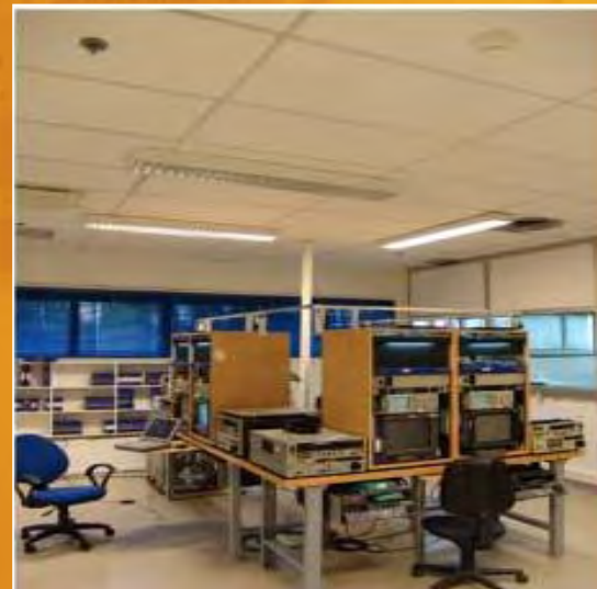
Smoke Detection & Sprinkler System
